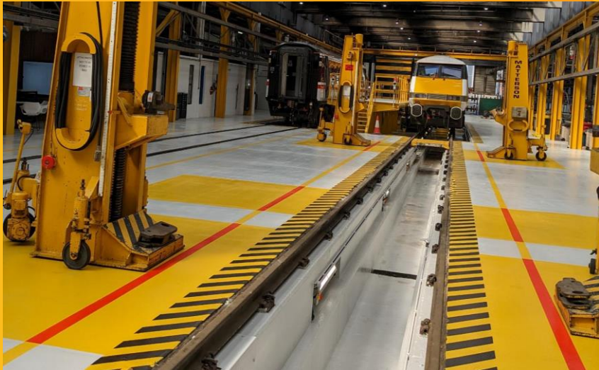
Power Car Bay at Neville Hill TrainCare Centre
