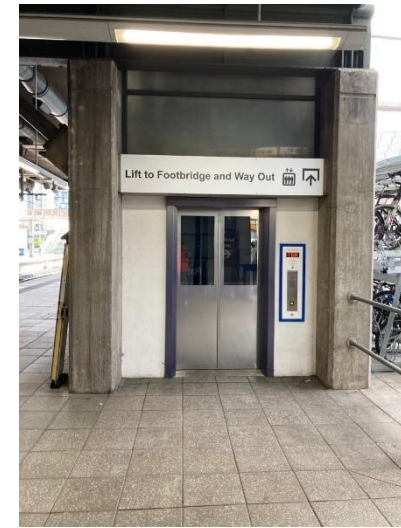
Figure 22: Lift access to platforms
